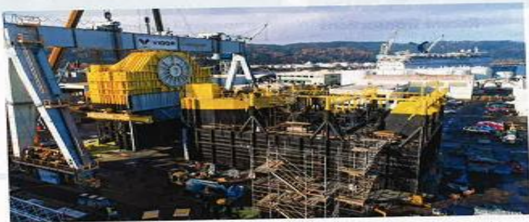
HAWAII BOUND Ocean Energy's Buoy will be towed from Portland, Ore., once construction is complete.
